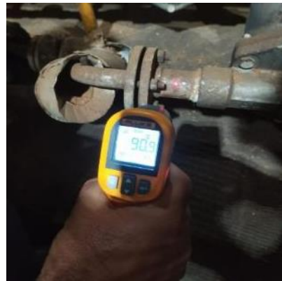
Scheduled Steam Trap Monitoring
